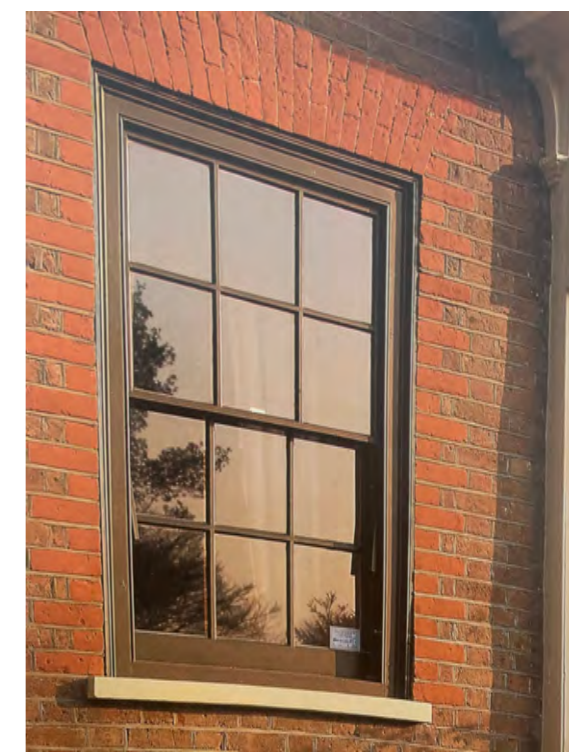
A dark brown coloured early sash window and frame sitting within orange/red brick dressings. (The Georgian Group)
